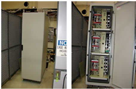
Fig. 7. Prototype 1 MW, 4160-V ac/1000-V dc converter.
